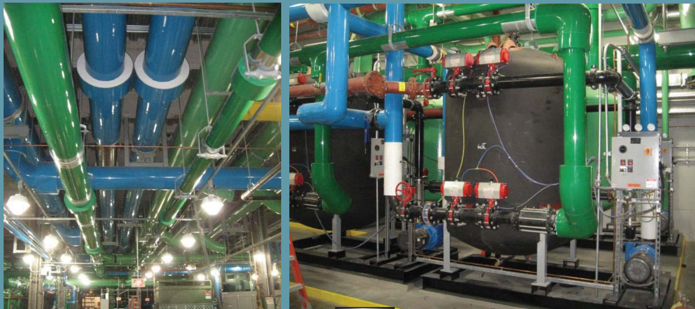
Cooling for 75 University buildings
