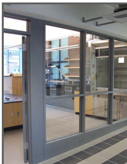
Jacobsen Lab Instrument Room (in new connector) Photo: JBM General Contractors, 2009
