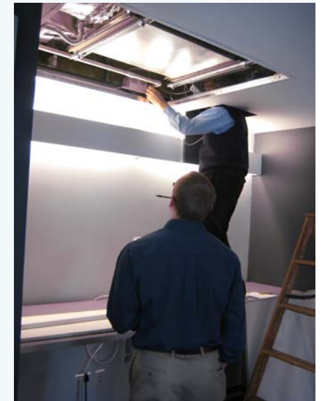
OFS and FMO commissioning the space
