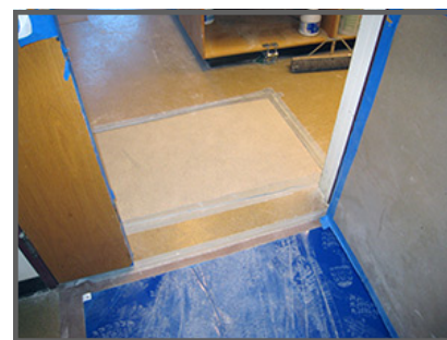
IAQ Management Housekeeping: Walk-off mats at entrance
